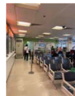
HEPA unit is placed at A&E area
