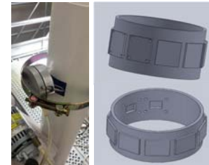
(Left) Sampling bioaerosol generated during flushing (Right) Ring-shape UV LED disinfection module for the drainage-ventilation pipe
