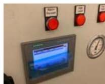
System Control Panel
