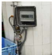
Electric & Water Meter
