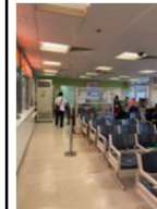
HEPA unit is placed at A&E area
